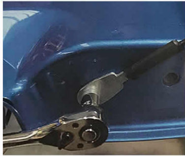
Tighten the tailgate strap bolt Do Not Overtighten as the cable needs to move freely
